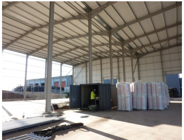
Progress at the Avonmouth energy recovery plant. The existing waste treatment facility can be seen in the background of the image above.
